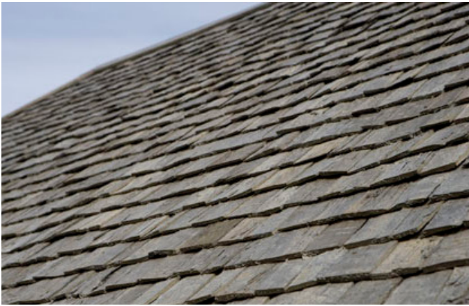
Norfolk Island Pine sourced for timber roofing shingles. Source: Department of Environment, 2007.
